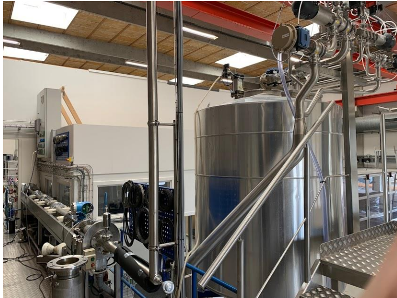
Figure 16: Medium sized flow rig at DTI, Denmark
