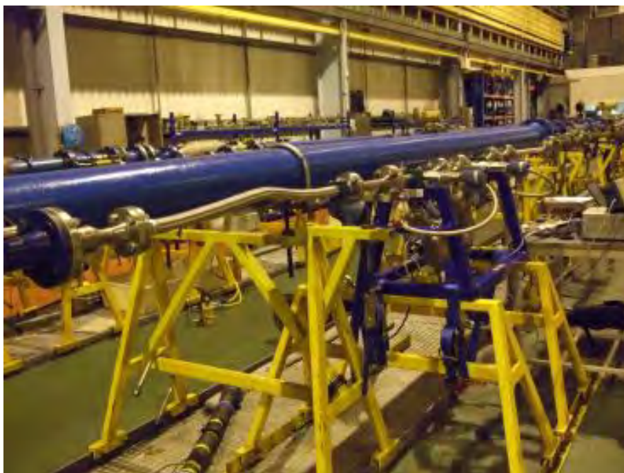
Figure 7 Installation in TUV NEL Oil Flow Line
