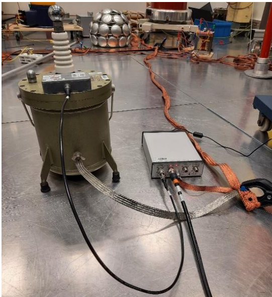
Figure 1. VTT voltage channel design: 20 kV gas-compressed capacitor and the active low-voltage arm.
